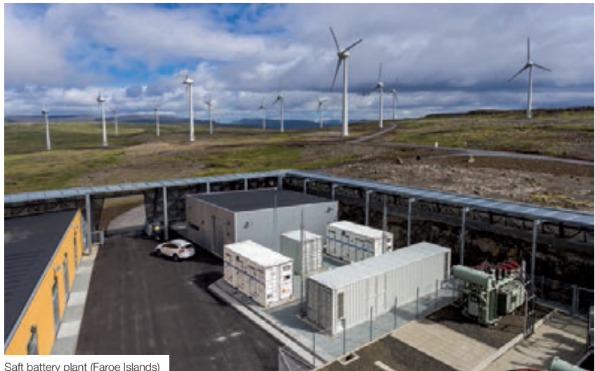
Saft battery plant (Faroe Islands)
