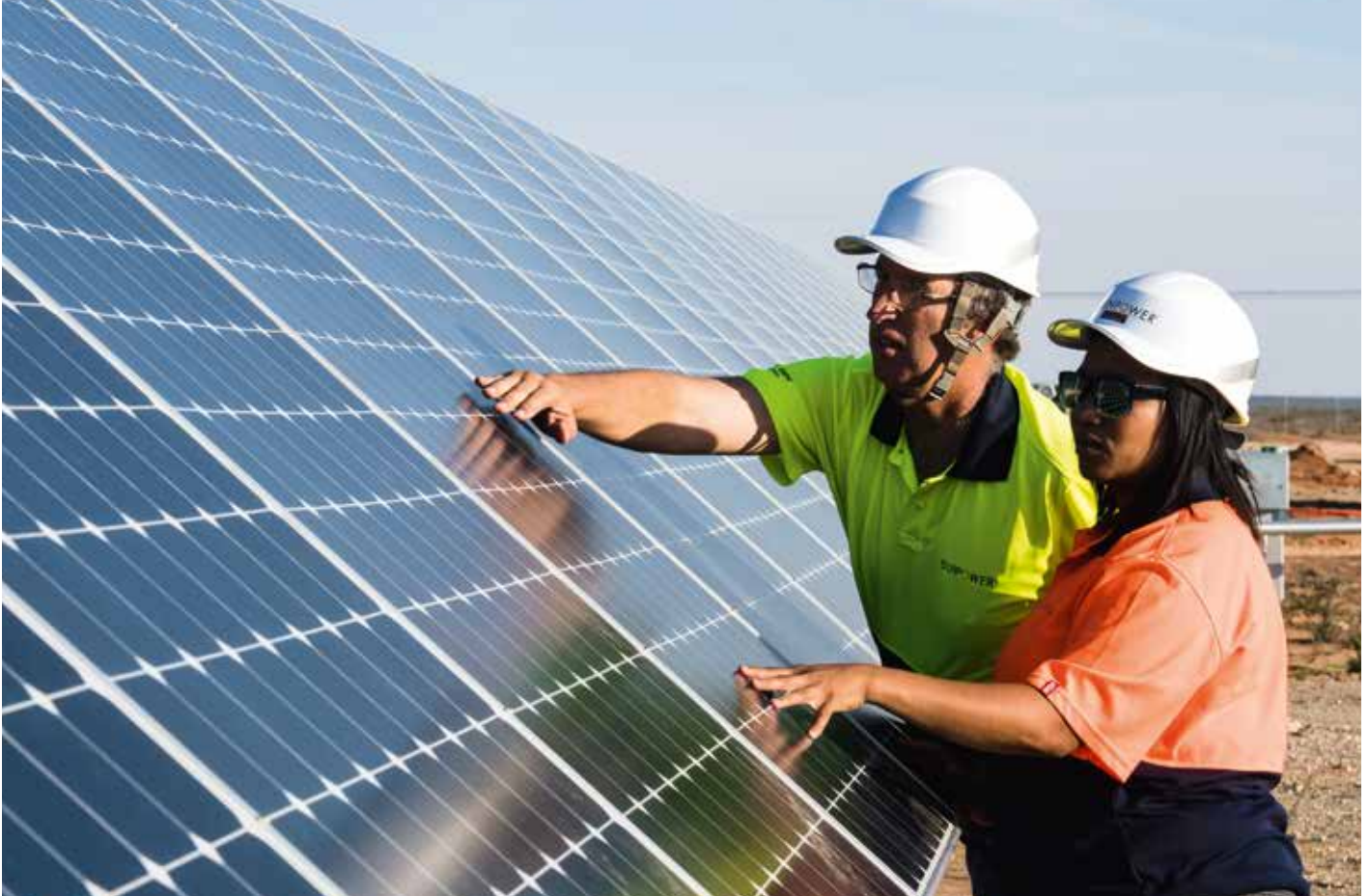
Operators at the Total SunPower solar power plant, Prieska, South Africa
